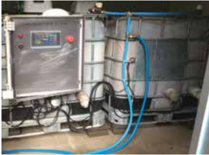
Dual IBC tote system (2000L combined capacity) dosing BiOWiSH™ Aqua into municipal STP raw inflow through a metering pump controlled by local PLC
