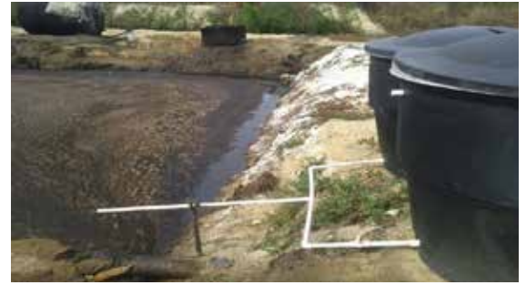
Dual tank setup (2000L combined capacity) drip dosing (gravity) through PVC tubing and spherical valves
